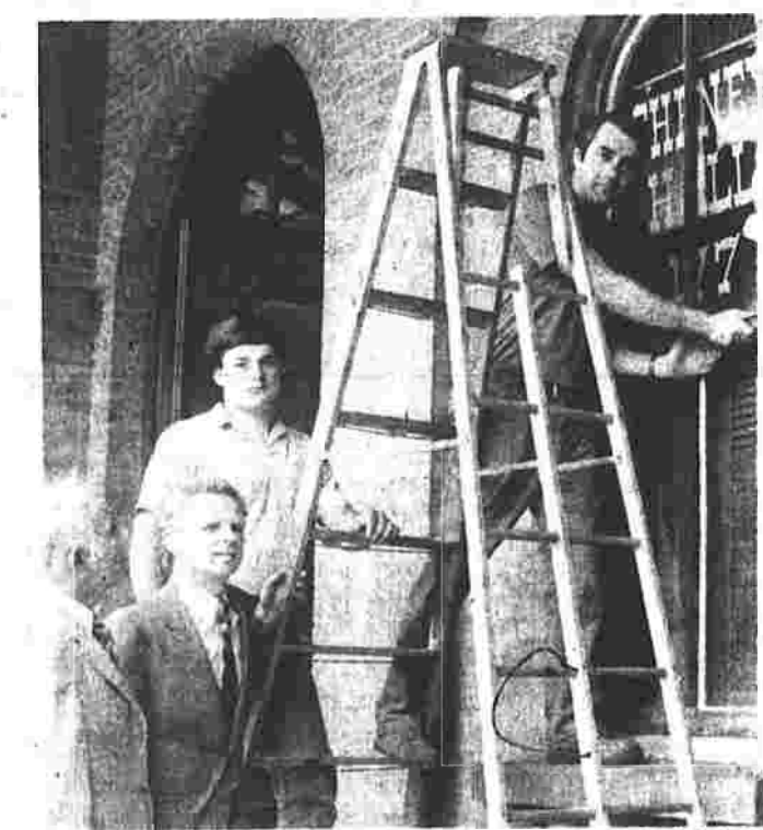
VOLUNTEERS HELP RENOVATE CHENEY HALL. From left, David Kahn, Bayer, White and Thomas
